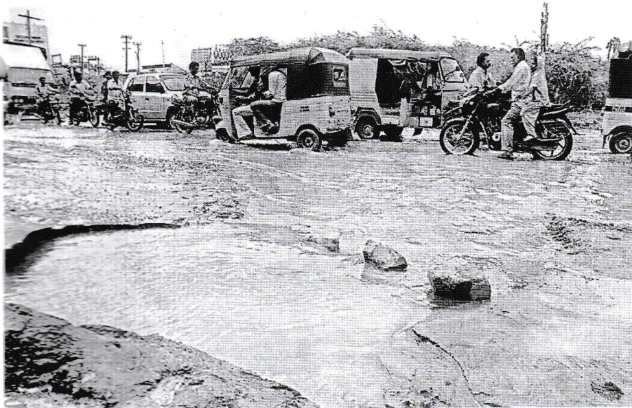
Metro water pipe broken in Ambattur, Chennai, India (Courtesy : Dinamalar)
